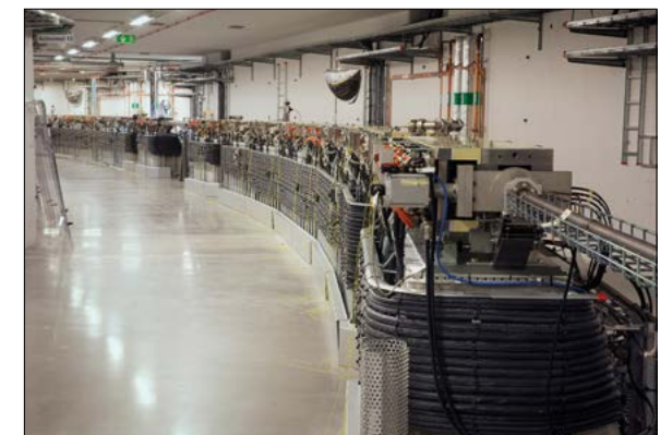
Part of the MAX IV 3 GeV ring showing iron-block magnets.
